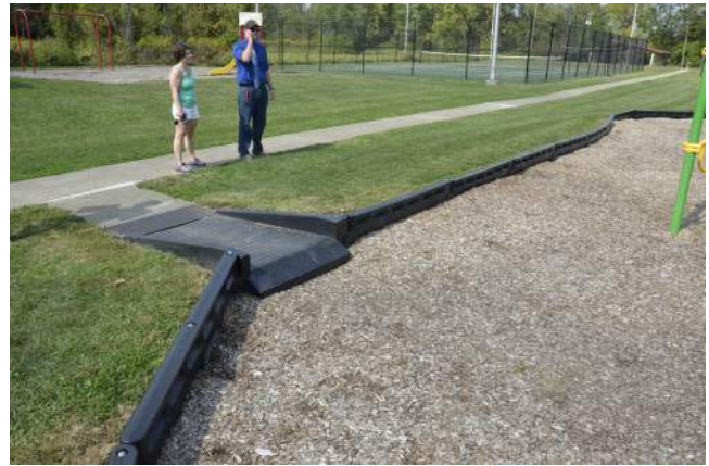
Figure 2.18: No accessible route to play area at Lions Park (2017).
