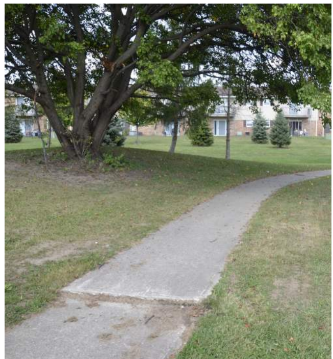
Figure 2.20: Potential trip hazard at National Road Park (2017).
